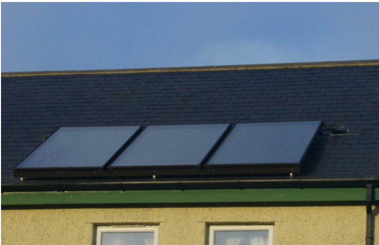
Above: showing three solar panels integrated with an air source heat pump
