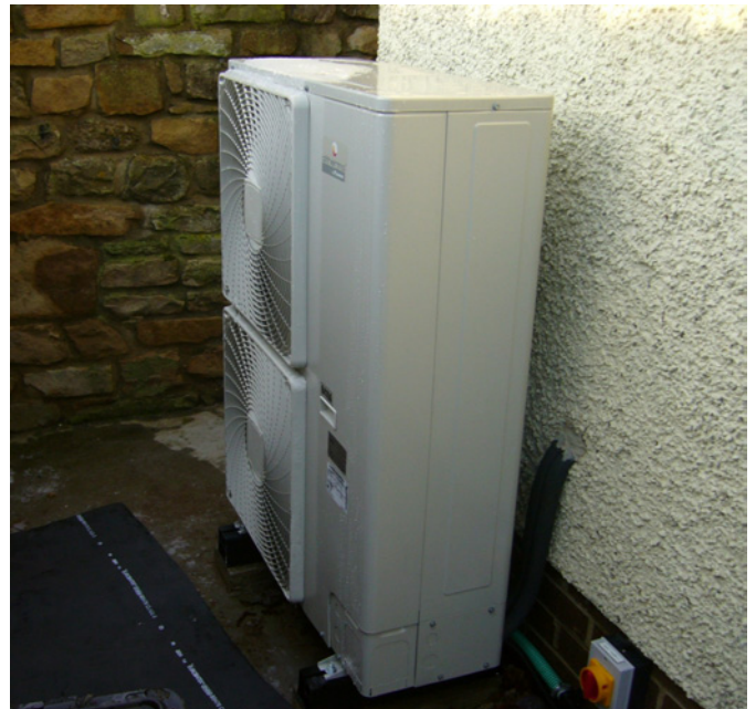
Above: showing the Daikin Altherma Air Source Heat Pump (outdoor unit)
