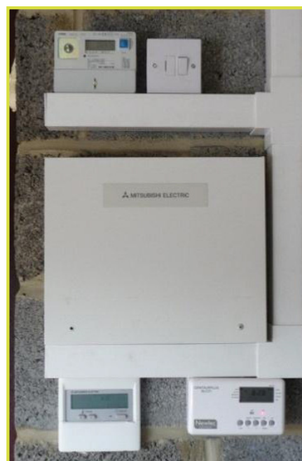
Above: Shows the renewable energy controllers
