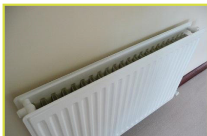
Left: Shows the renewable energy working throughout the house by heating the radiators
