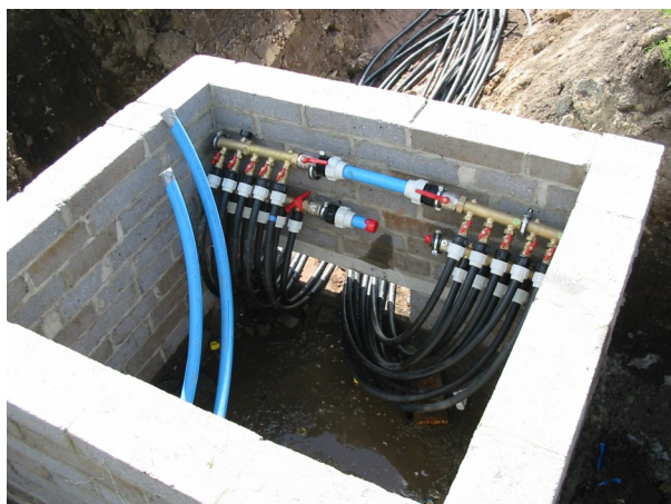
Above: showing the manifold chamber where all the ground pipes are connected up to the manifold and then feed to the flow and return pipes (in blue) to the heat pump.
