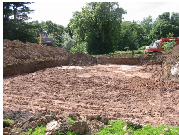
Above: a cleared area 1.2m deep with the pipe work installed and covered in sand to protect the pipes.
