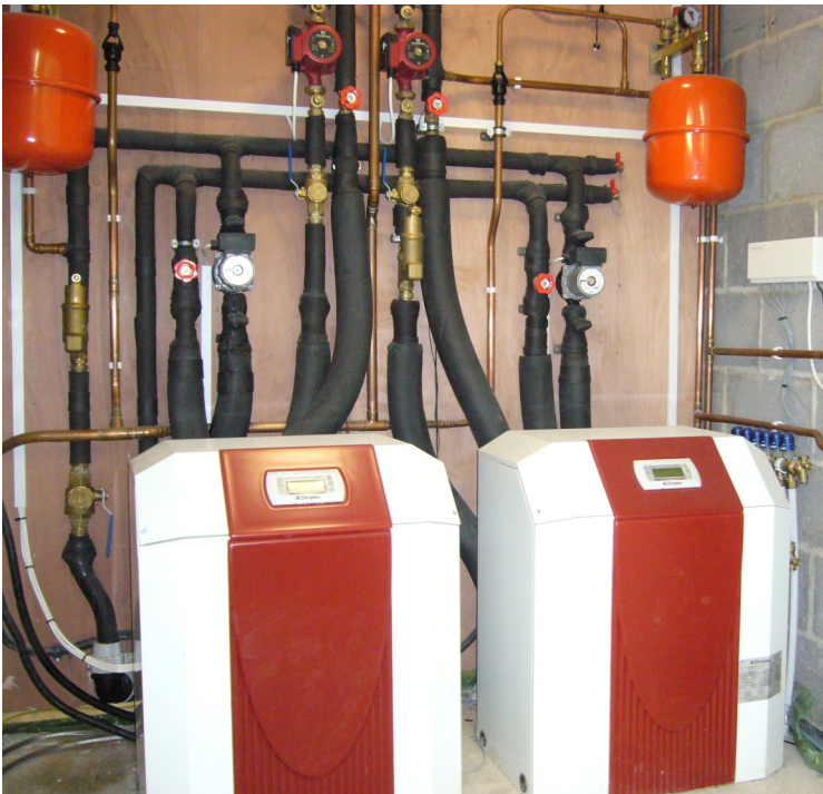
Above: shows the complete installation of the Dimplex 22kW set in the boiler room.
