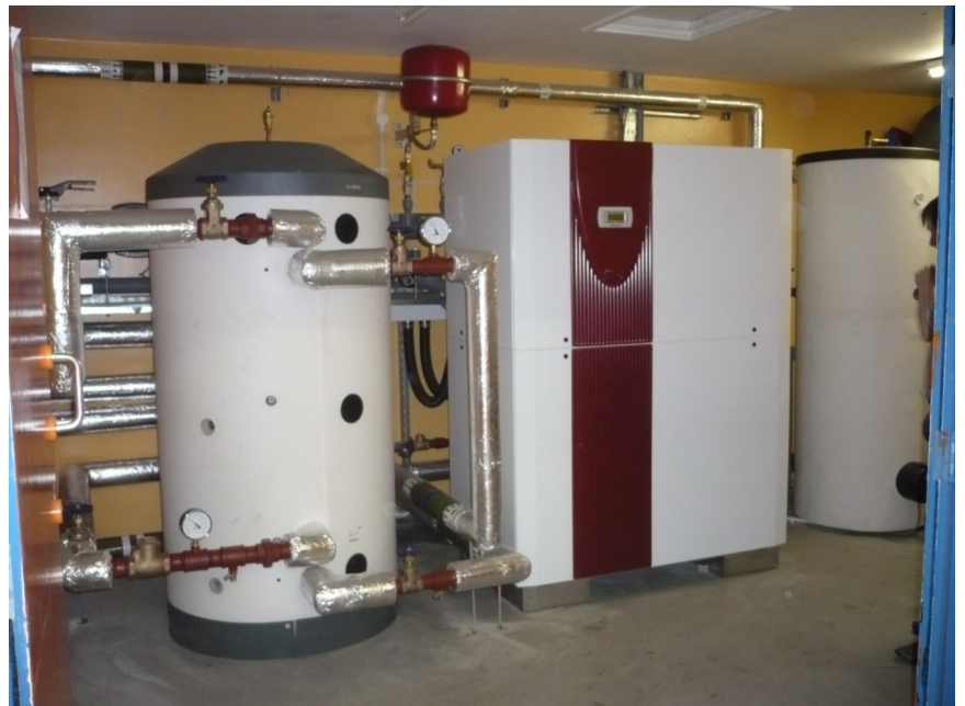
The above picture is the installed Dimplex 50KW Ground Source Heat Pump with hot water cylinder and a solar buffer tank.
