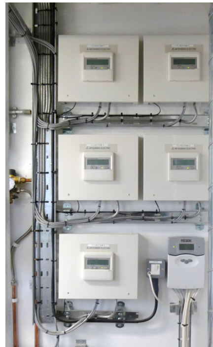
Above left: Plant room showing 1800L thermal storage for the renewable energy systems
